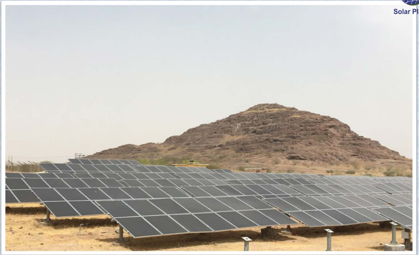
Solar Park at Jodhpur
